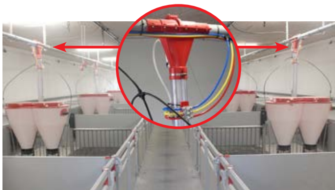
COLOR FEED SINGLE: Phase feeding valve in a weaner unit
